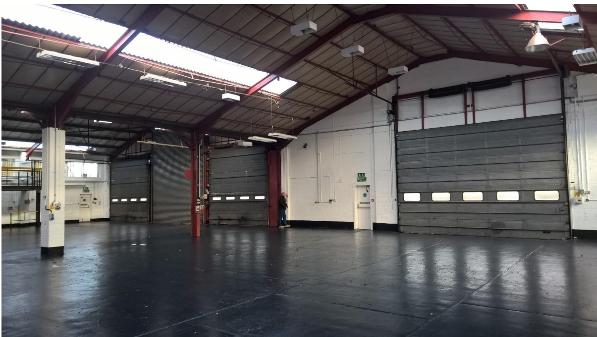
Figure C2 – Photograph inside the main transfer station building, illustrating the block walls and the sound integrity of the doors and roof.
